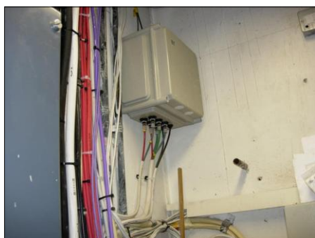
PHOTOGRAPH 13 EXISTING BT FIBRE SPLICE ENCLOSURE IN RISER CUPBOARD ON FIRST FLOOR LANDING
