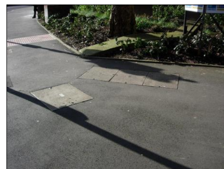
PHOTOGRAPH 3 EXISTING BT AND VIRGIN MEDIA CHAMBERS IN FOOTWAY ADJACENT TO BUILDING FRONT ENTRANCE
