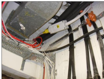
PHOTOGRAPH 11 EXISTING BT FIBRE SERVICES IN RISER CUPBOARD IN RECEPTION ON GROUND FLOOR
