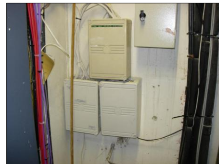
PHOTOGRAPH 12 EXISTING BT COPPER SERVICES IN RISER CUPBOARD ON FIRST FLOOR LANDING
