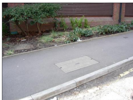
PHOTOGRAPH 1 EXISTING BT CHAMBER IN FOOTWAY ON WARWICK ROAD SERVICING BUILDING
