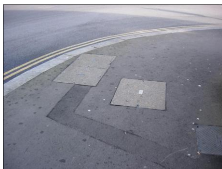
PHOTOGRAPH 5 EXISTING BT AND VIRGIN MEDIA CHAMBERS IN FOOTWAY ON QUEENSWAY OPPOSITE BUILDING
