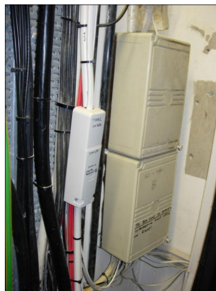
PHOTOGRAPH 14 EXISTING BT COPPER AND FIBRE SERVICES IN RISER CUPBOARD ON SECOND FLOOR LANDING
