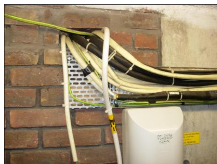
PHOTOGRAPH 8 EXISTING BT CABLE EXIT LOCATION AT HIGH LEVEL FROM INTAKE ROOM TO CAR PARK AREA
